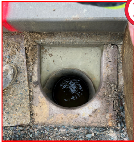
Gully set too far away from kerb.
