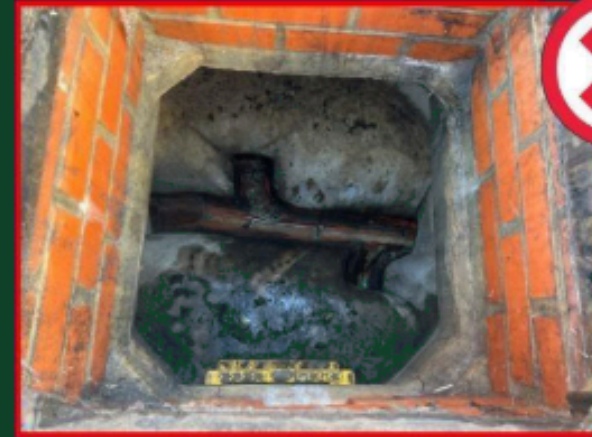
The brickwork is laid to the wrong bond.
