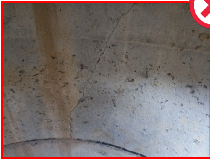
Crack in ring.
