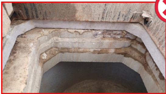
Raisers misaligned, lid and top raising section dry-bedded and damaged
